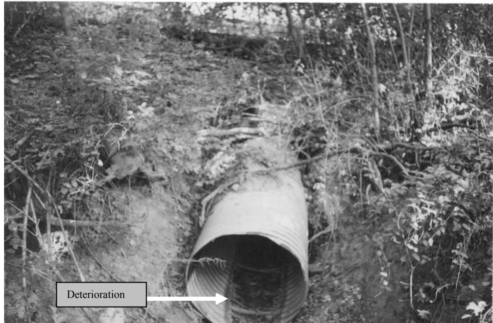
Figure 5–28. Culvert and gully with Rayloc Drive above. Note culvert dropped below original horizontal plane and rusted.
